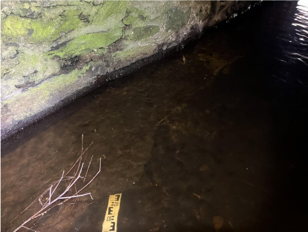
Photograph B-29 – View of the scour and undermining at the south end of the structure
