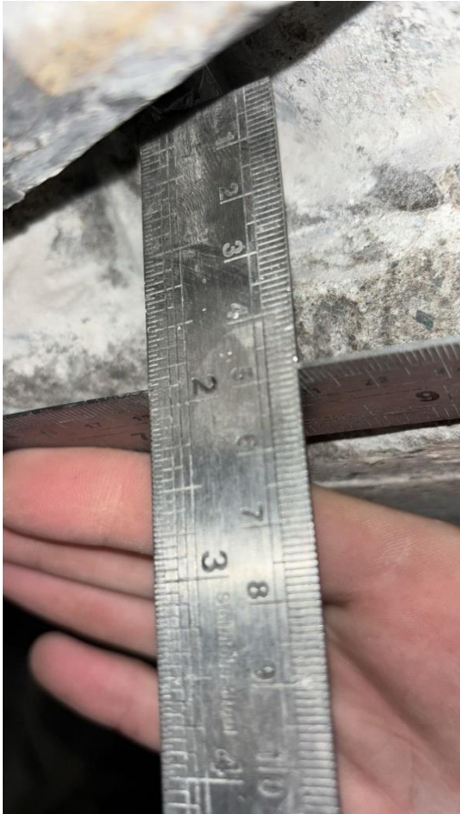
Area 4 Transverse smooth rebar 48mm cover
