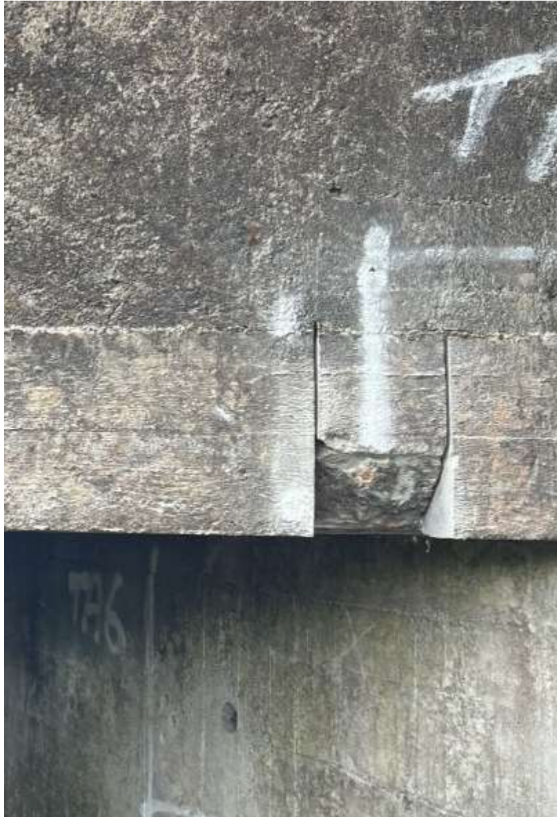
Figure 18: No reinforcement found in the breakout
