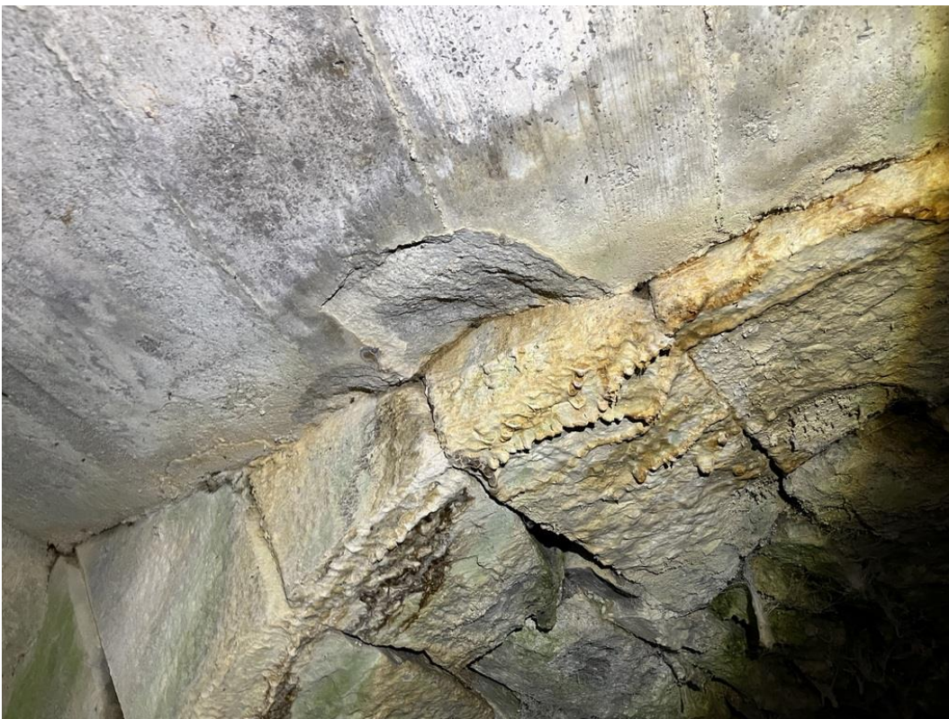
Photograph B-26 – View of the spalling to the concrete deck at the south end of the deck (Area 3)
