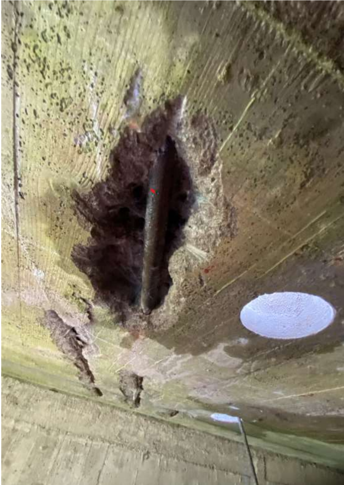
Figure 22 : Breakout area with core holes C1,C2 to the right
