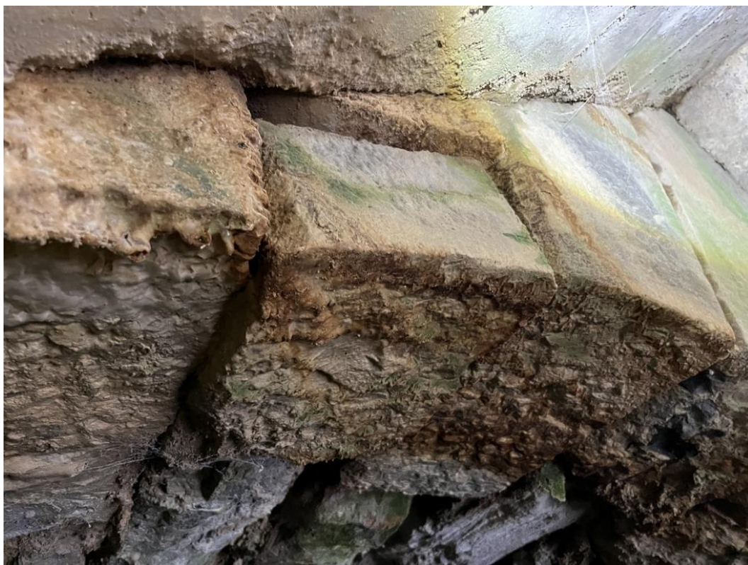
Photograph B-21 – View of the cracked voussoir stone at the northern end of the arch barrel
