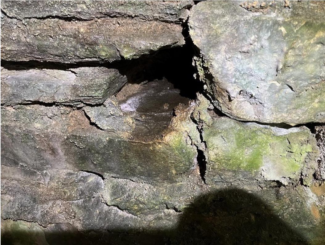
Photograph B-19 – View of the missing masonry to the arch barrel (Area 2)
