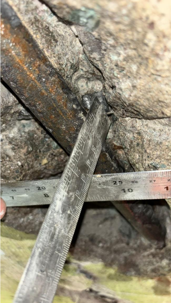
Area 3 transverse smooth rebar 43mm cover
