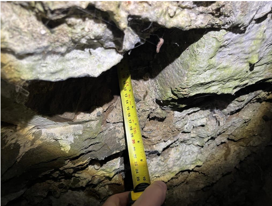
Photograph B-20 – View of the missing masonry to the arch barrel (Area 3)
