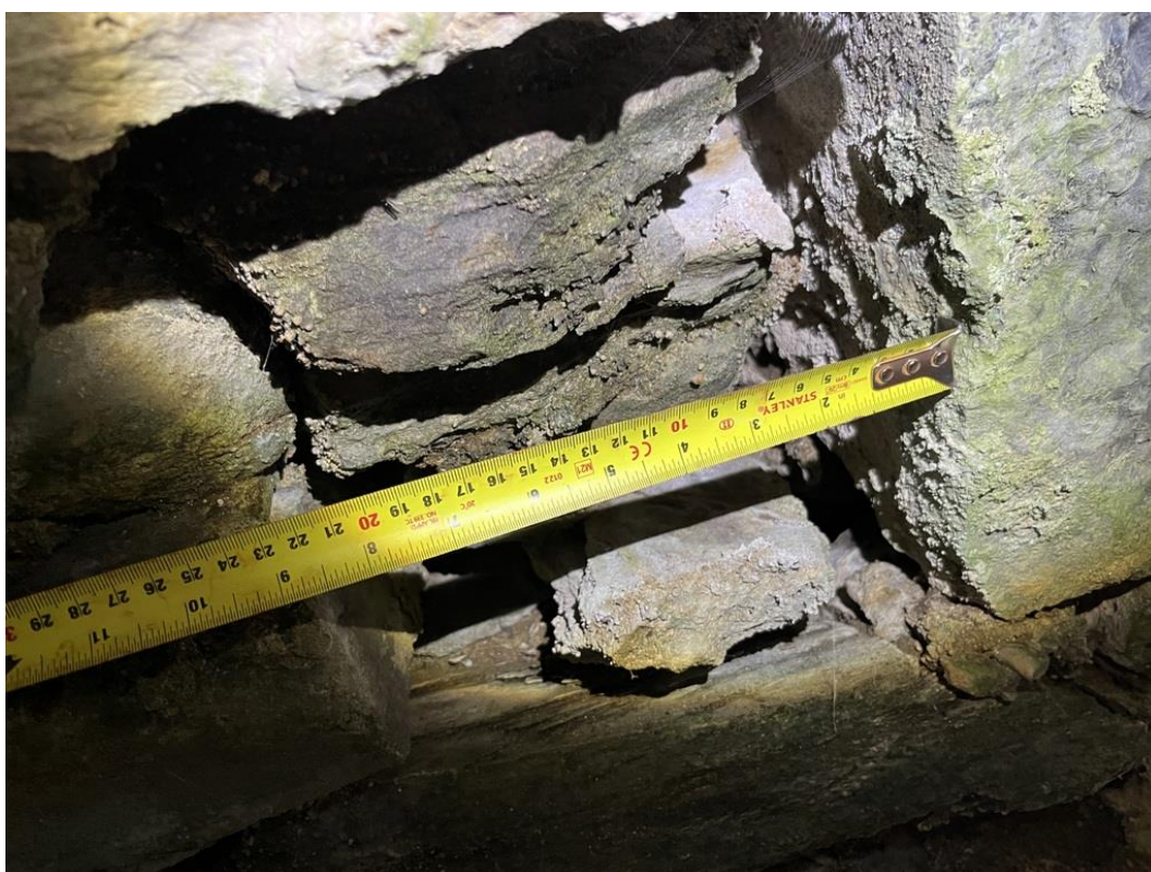
Photograph B-18 – View of the missing masonry to the arch barrel (Area 1)
