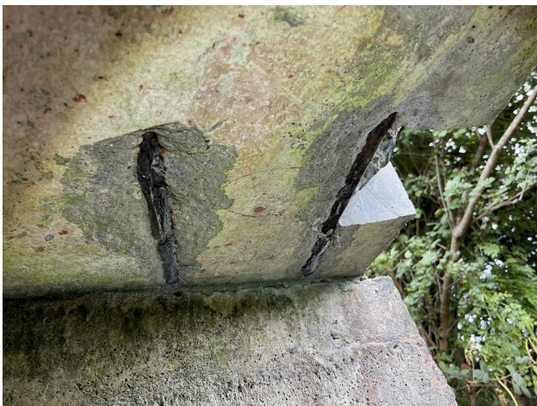
Photograph B-24 – View of the spalling to the concrete deck at the northern fascia (Area 1)
