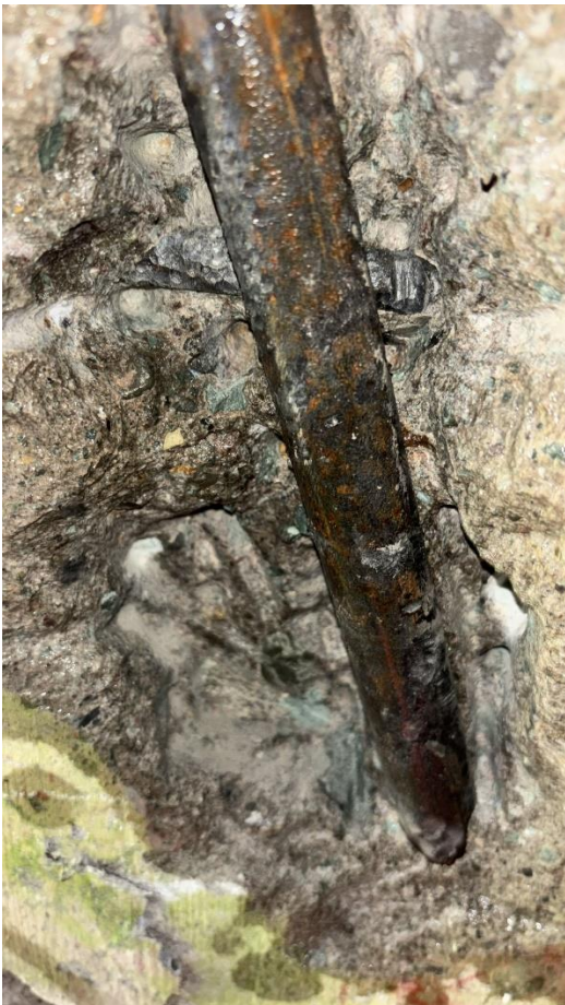
Area 3 Soffit breakout
