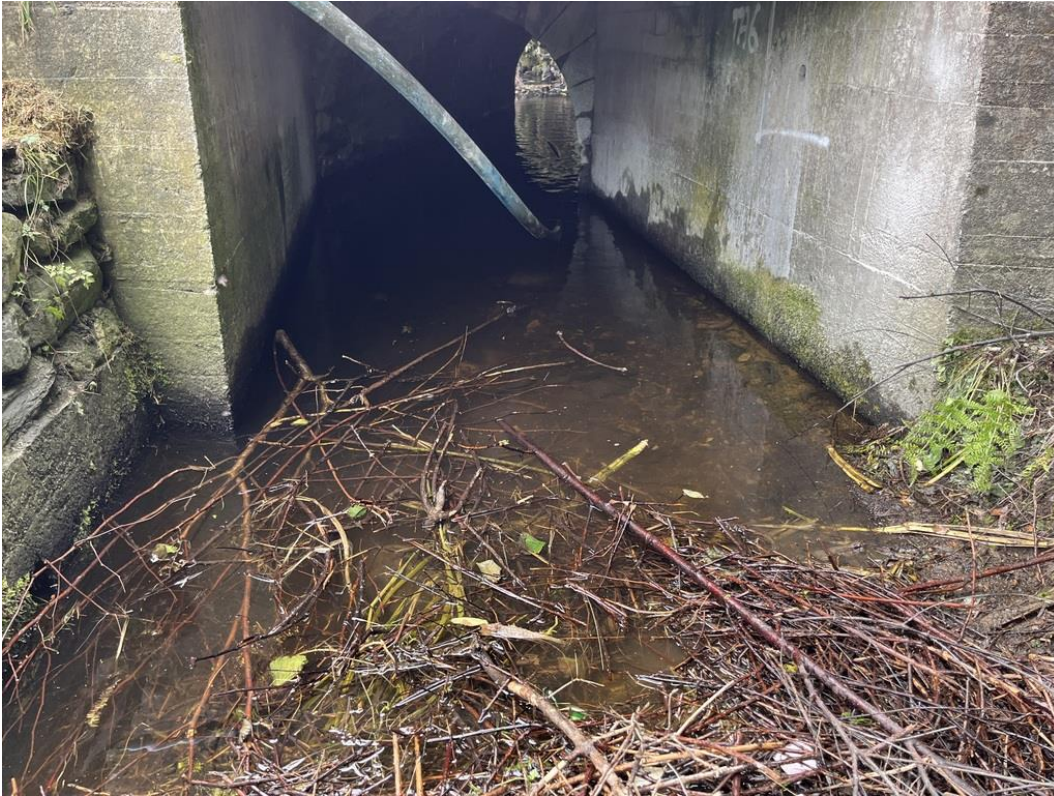
Photograph B-27 – View of the river at the north elevation with debris evident
