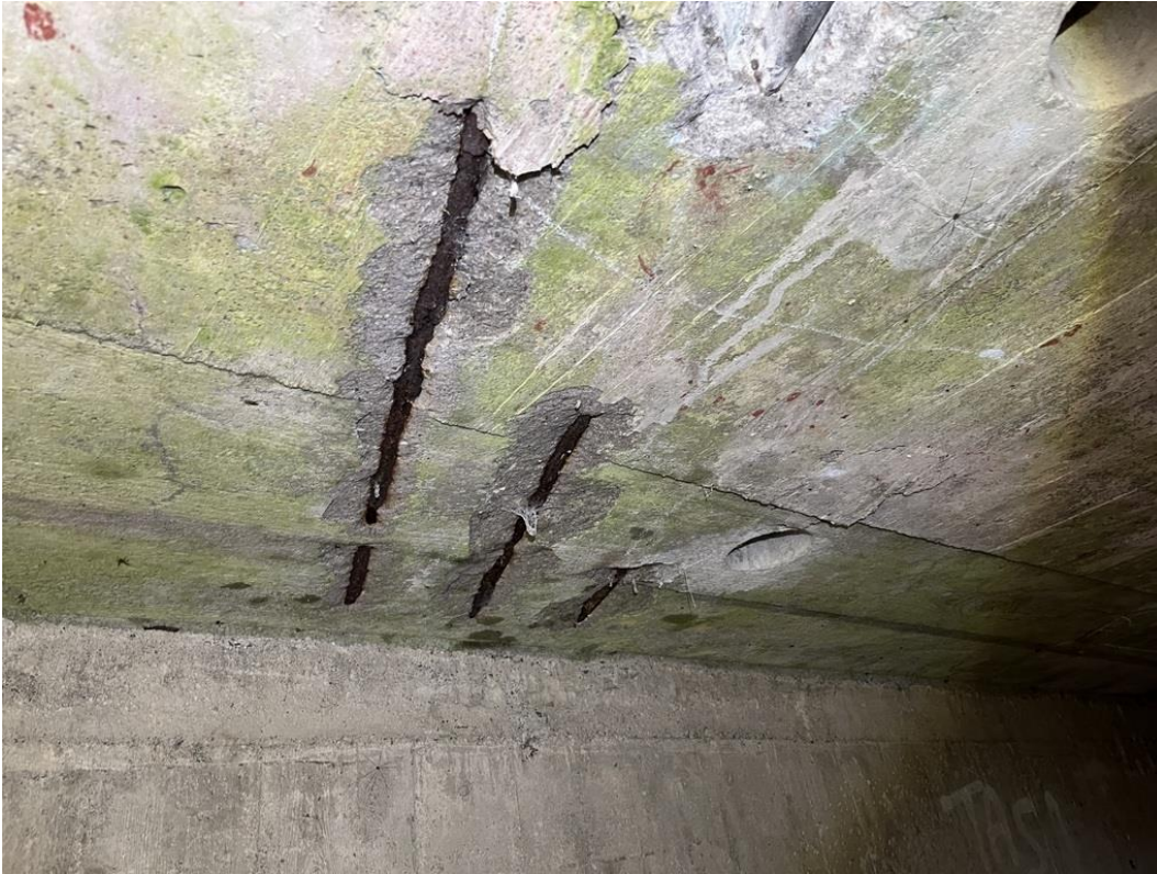
Photograph B-25 – View of the spalling to the concrete deck 0.8m from the north elevation (Area 2)
