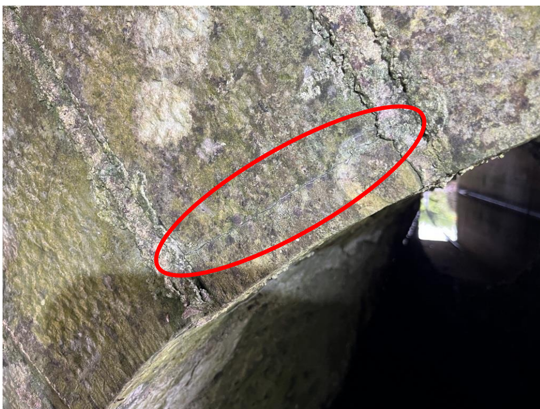
Photograph B-22 – View of the cracked voussoir stone at the south elevation
