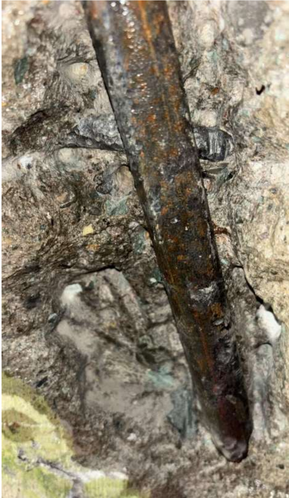
Figure 23: Close up of exposed reinforcement
